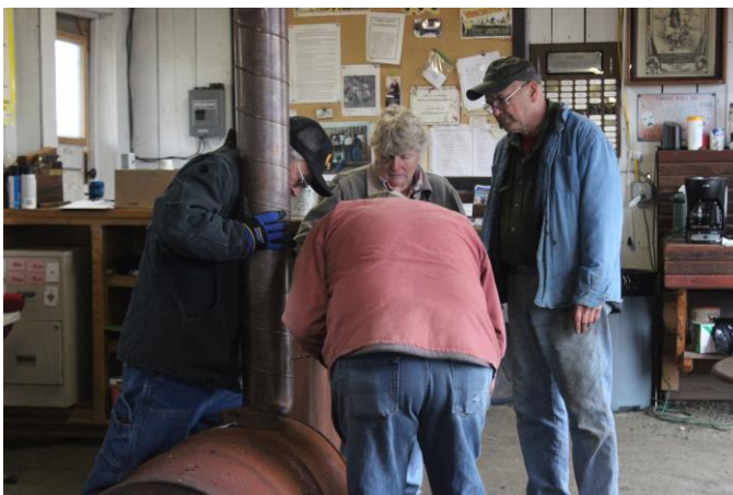
Covada oversees Crazy Knife & Del Monte installing the damper while Granny looks on.
